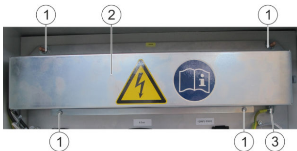
Fig. 26: High voltage generator cover
