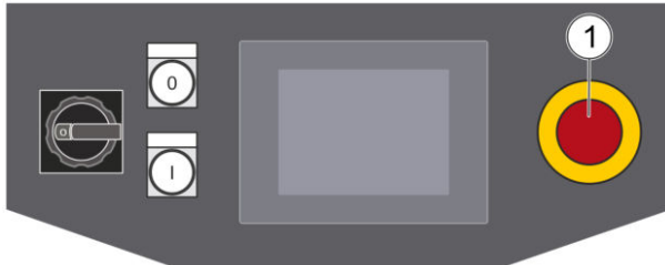
Fig. 5: Emergency stop button
